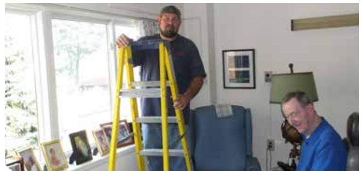
Mike Gaggy from Honeywell installing Resident Council V.P. Bob Riley's new unit.
